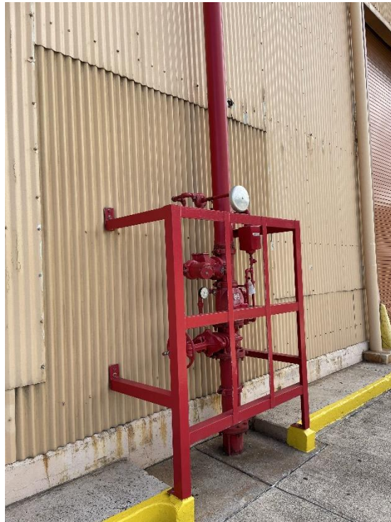
Photo 4: Example of new fire suppression system.
